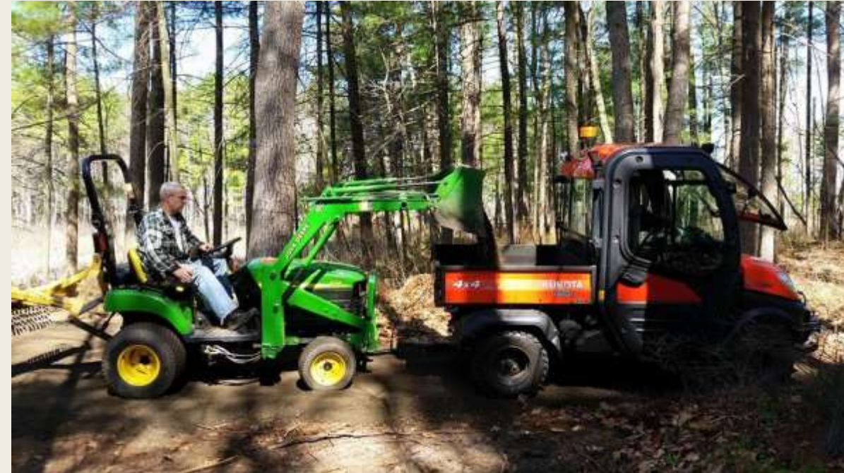
Member using his personal tractor to load the Kubota with material to address erosion issues.
